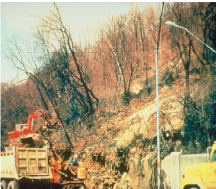
A highway crew removes material along the Columbia Parkway in Cincinnati, Ohio. Leaning trees are an important indicator for unstable ground. Photography by Bob Fleming, USGS.
