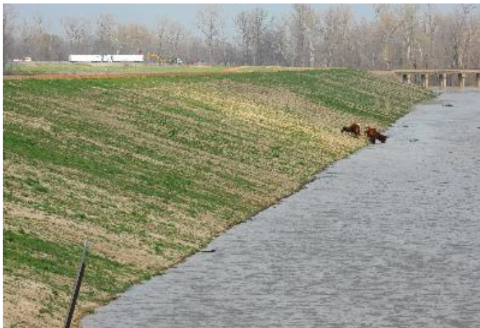
A levee in West Memphis, Arkansas. Photo by Jocelyn Augustino and courtesy of FEMA.
